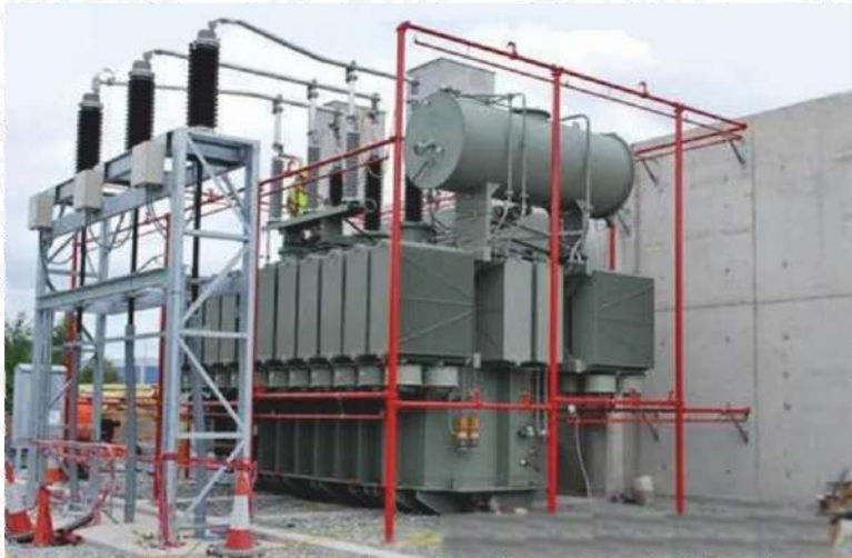
OFF (WORKING) WATER SPRAY SYSTEM
