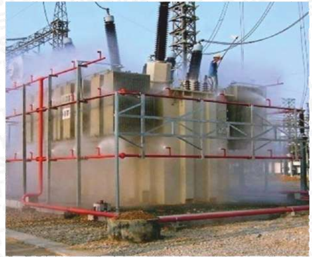
ON (WORKING) WATER SPRAY SYSTEM
